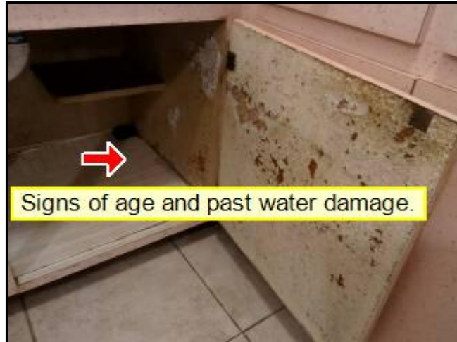
1.5 Picture 2 Moisture damage.
